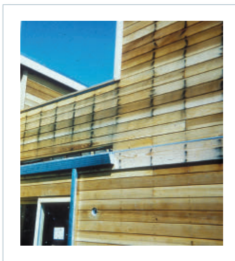
Figure 8 —Iron stain on newly constructed home. The intent of the owner was to have a natural finish (lightly pigmented semitransparent stain) on the siding. To correct this, the siding will need to be replaced.
