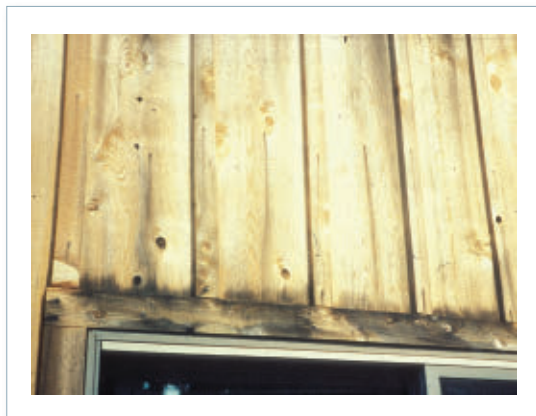
Figure 3 —Extractive bleed from end-grain absorption of water. Note the fasteners have also caused iron staining.
