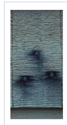
Figure 7 —Iron stain around electro-plate galvanized fasteners.
